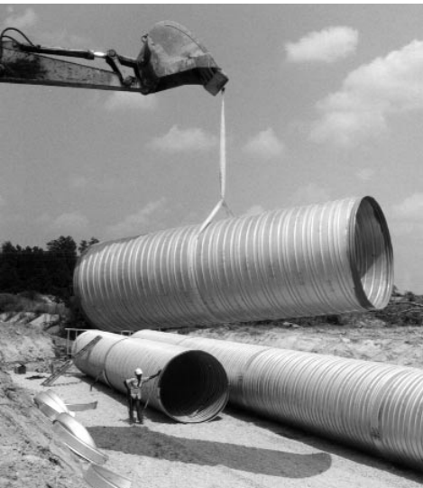
A section of corrugated steel culvert pipe is installed at a highway project.
